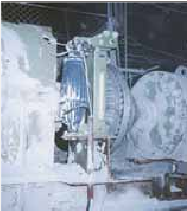
Kali und Salz AG, Unterbreitzbach works, conveyor drive, disk brake RST 2 with ELHY version EB 1250 – 60 Lm 2
